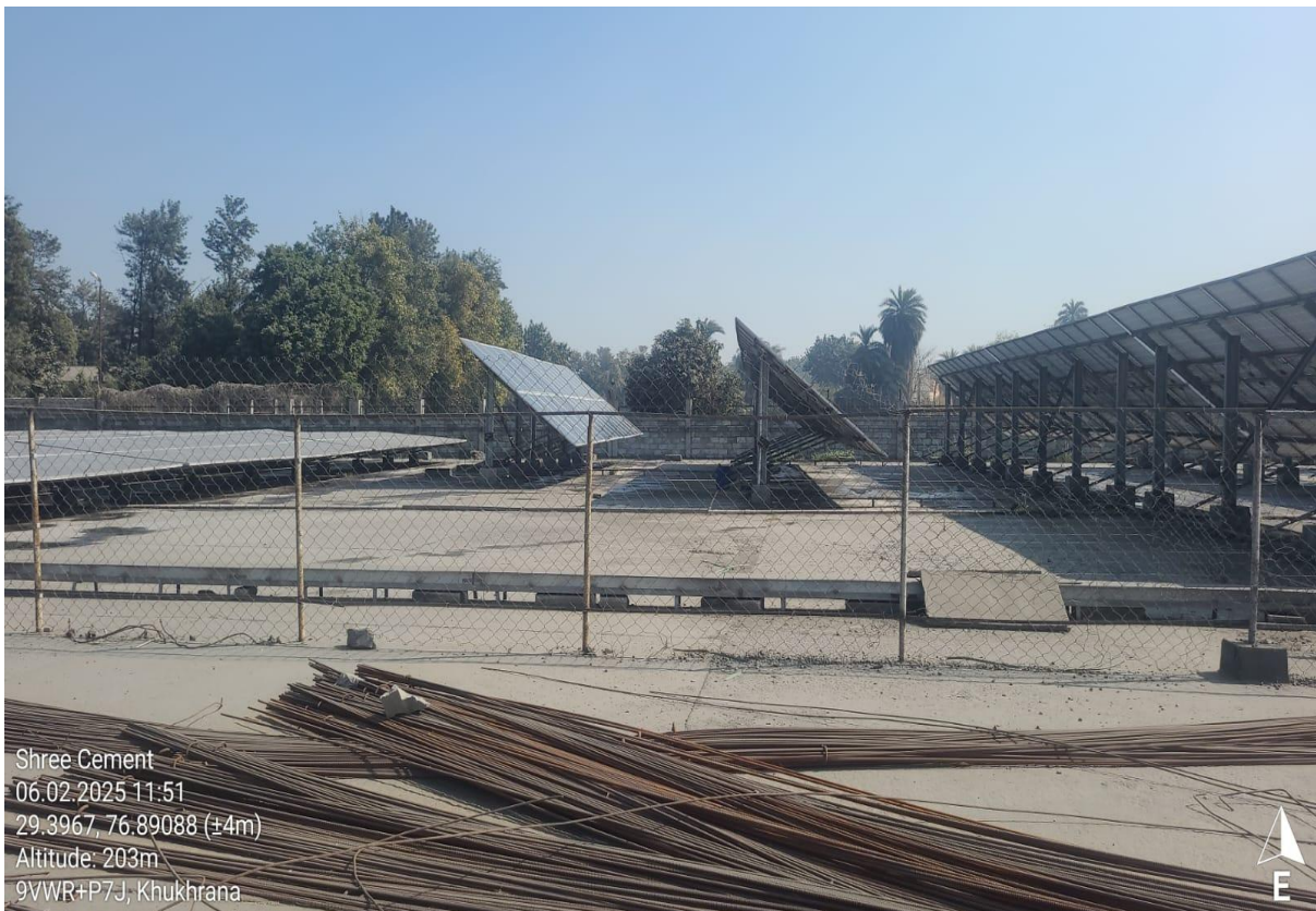
Photograph 8: Solar Power Plant
