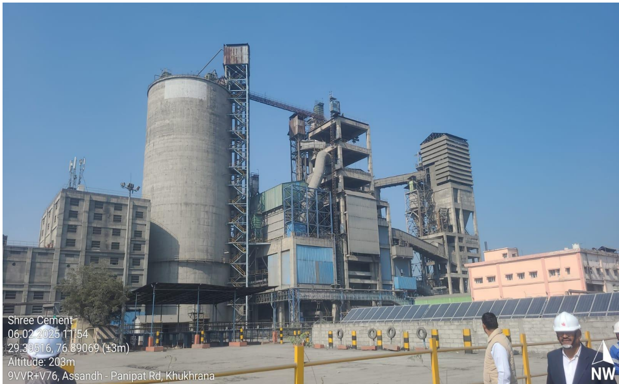
Photograph 1: Silos with bag filters
